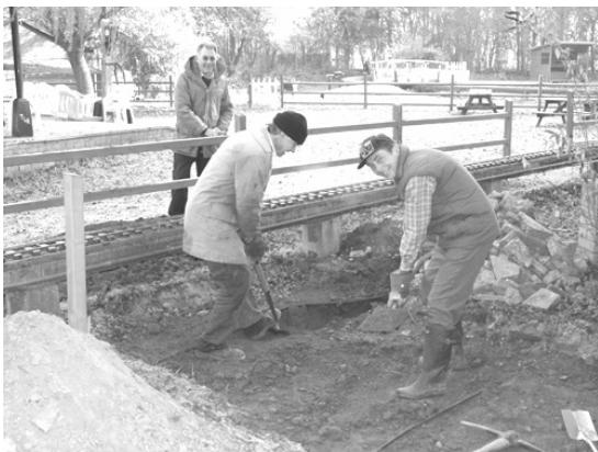
Movement of raised track rolling stock will be facilitated by the completion of these extensive earthworks.
