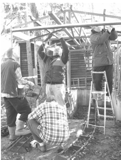
Slow but sure progress is being made on the ground level railway structures.
