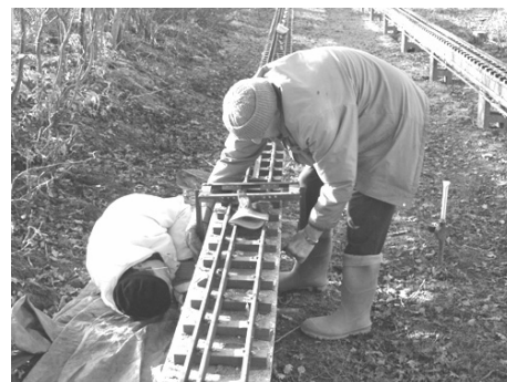
Work continues on installation of important anti-tip rails around the raised track
